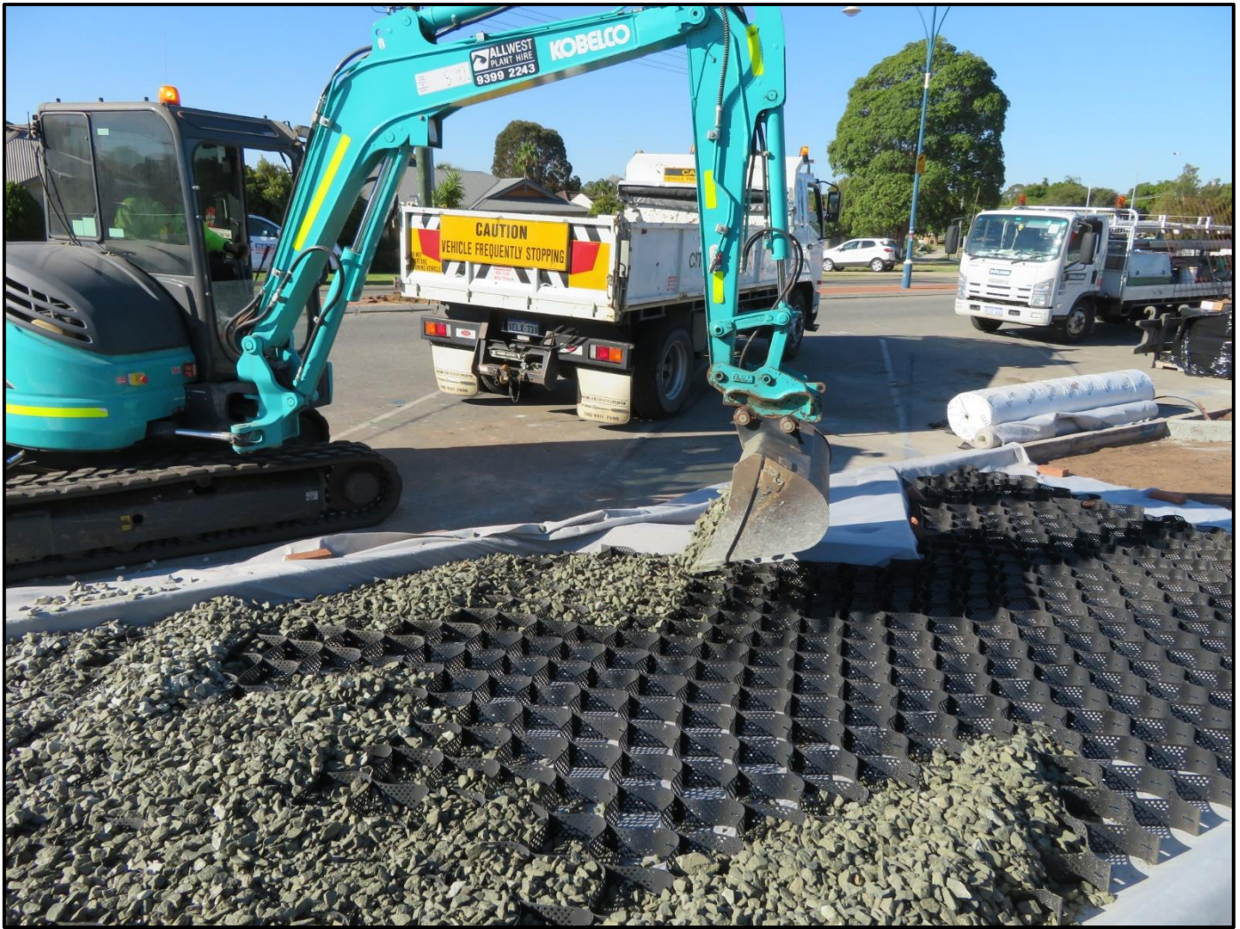
Figure 9. Example of GeoWeb product being installed within Epsom Avenue, Belmont – Image source City of Belmont (WA)
